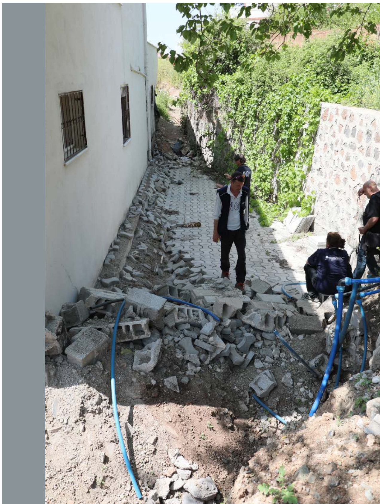
Photo 36 (37.490882°N, 37.067873°E) – At this site (view from the northeast) the coseismic rupture trace runs parallel to the house wall uplifting the house with respect to the paved outdoor, no clear significant damage can be reported.
