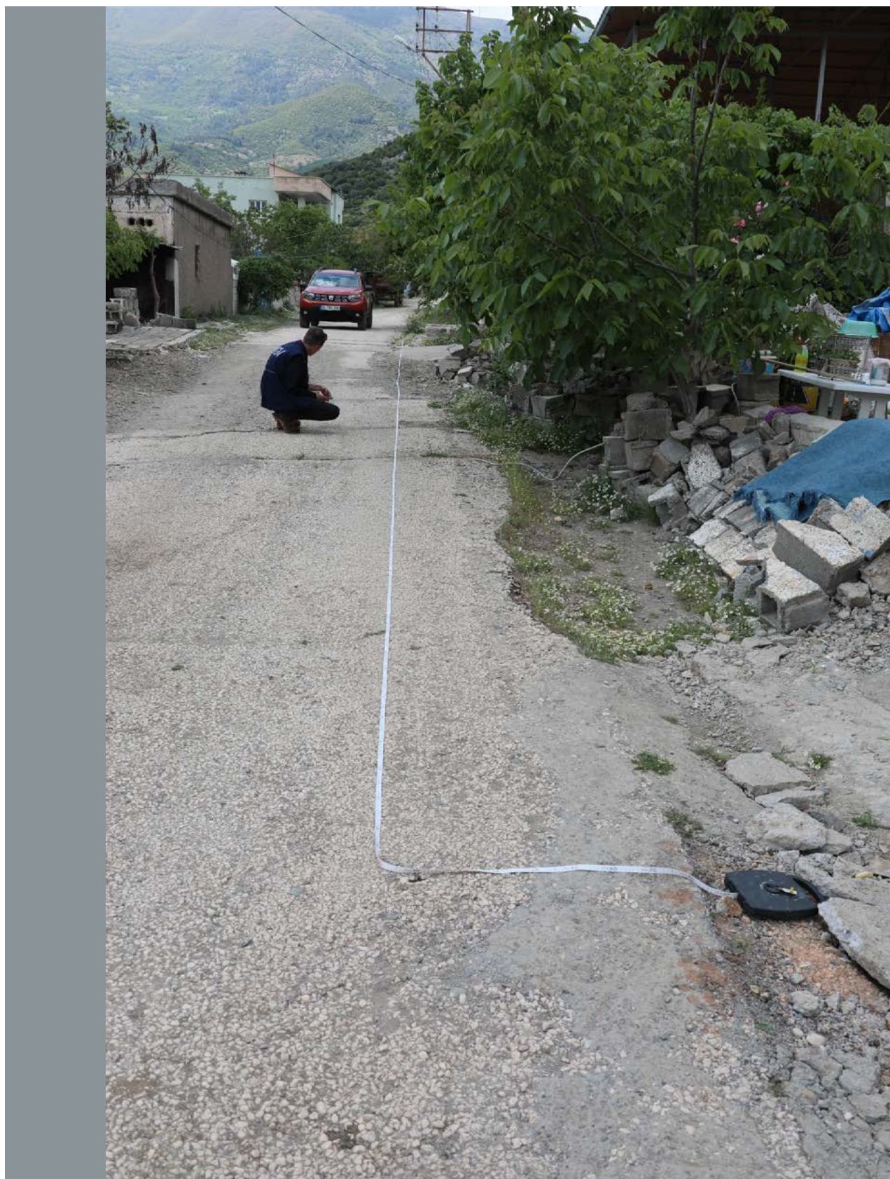
Photo 1 (37.127789°N, 36.667270°E) – The fault trace runs through the village of Kozdere (Islahiye district, Gaziantep province), offsetting roads with more than one meter of displacement. Although repairs restored most of the infrastructure affected by the faulting, its surface traces were still documented throughout the village. Here, a clear example of a tar road displaced by distributed deformation, which as a whole exhibits a purely left-lateral net offset of 90 cm.
