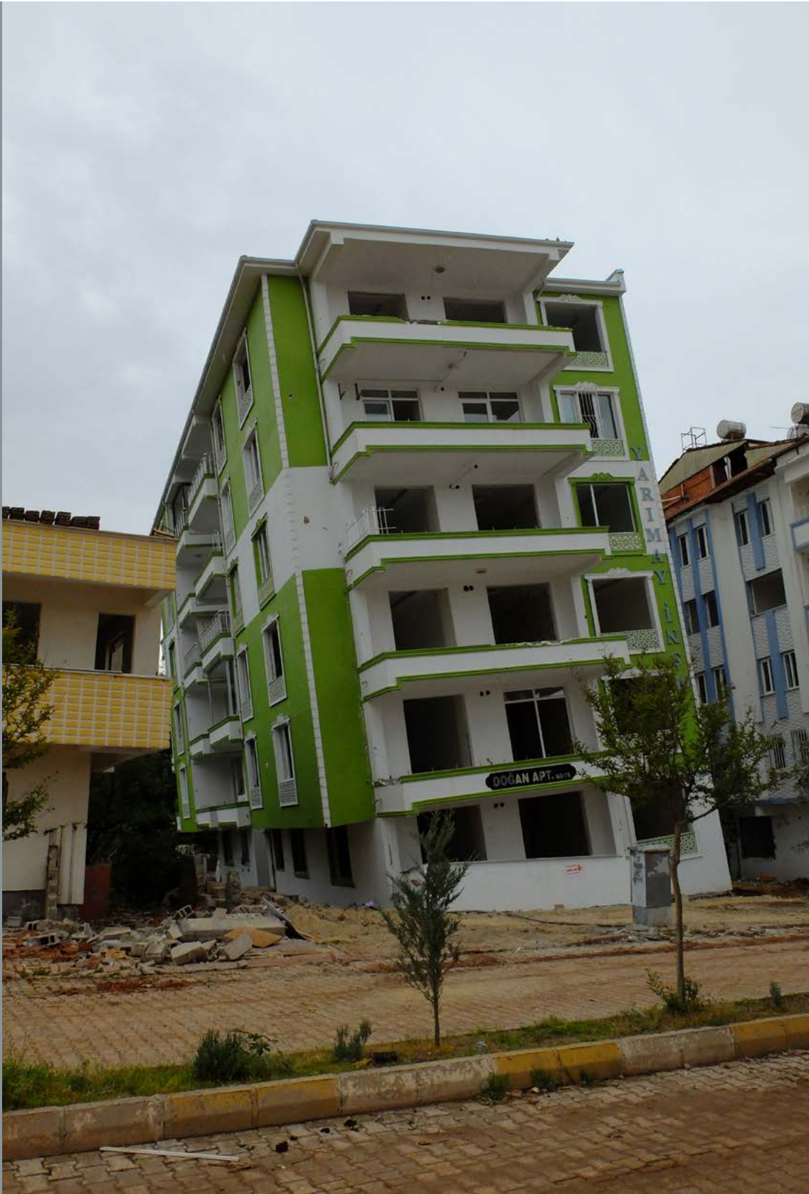
Photo 114 (37.788786°N, 37.645323°E) – Detail of the previous photo showing the differential settlement caused by liquefaction effects under the structure's load, resulting in severe tilting of the building.
