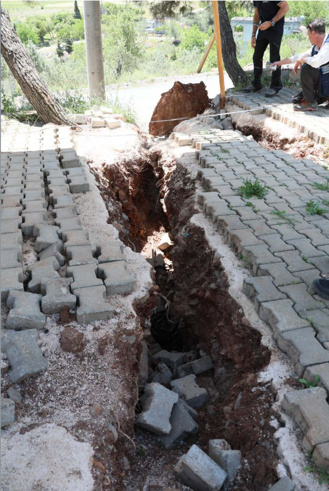
Photo 14 (37.164370°N, 36.706508°E) – Detail of the previous photo 13 (viewed from the north). The coseismic surface rupture is characterised by two en-echelon, decameter-scale transtensional branches with a large opening component and a meter-scale interposed gravity graben.
