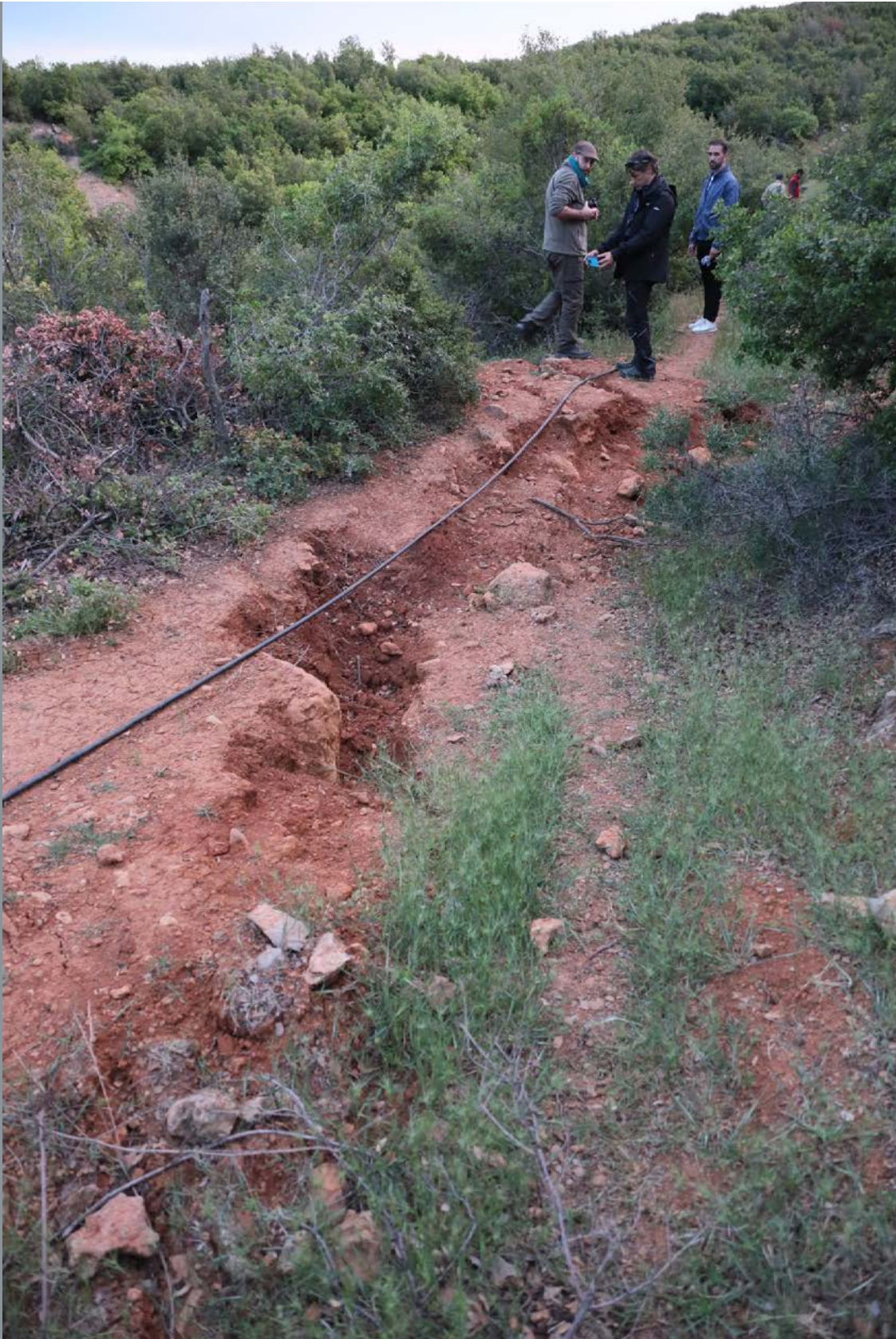
Photo 4 (37.139790°N, 36.679613°E) – Coseismic surface rupture highlighted by a mole-track with a pressure ridge, approximately 8 m in length, showing up to 70 cm of vertical component of the deformation.
