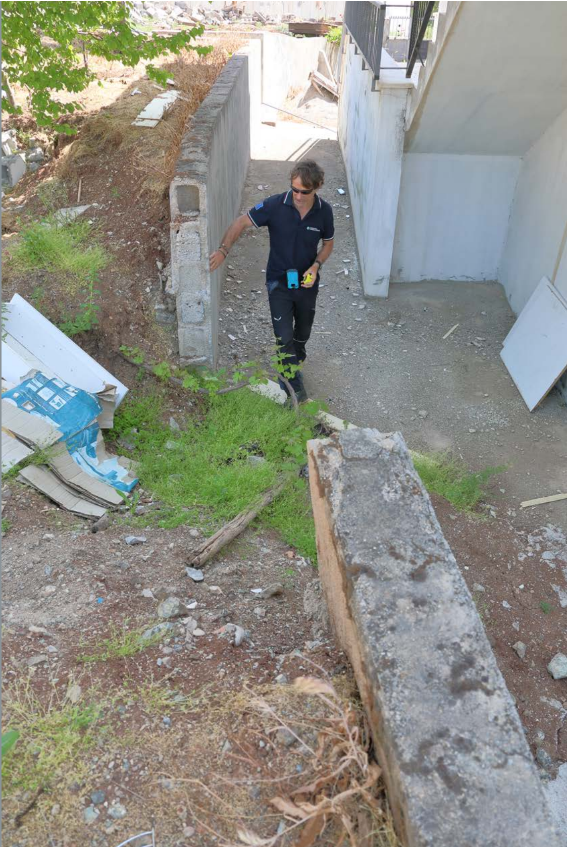
Photo 35 (37.490467°N, 37.066978°E) – Retaining wall in the Çiğli village affected by coseismic surface faulting displaying a pure left-lateral offset of 260 cm.
