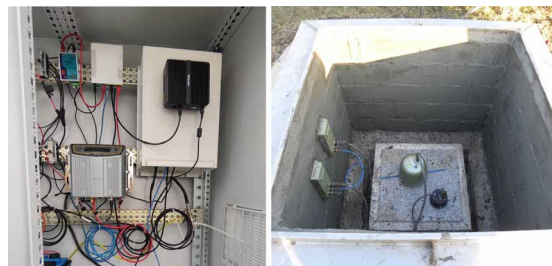
Figure 7 On the left the photo of the new installation of the PSB1 station where it is possible to see the mini-PC (black device) installed on the Nanometrics Cygnus system, on the right the photo of the sensor well where the Trident digitization system and the two seismic sensors are installed, the velocimeter and the accelerometer.
